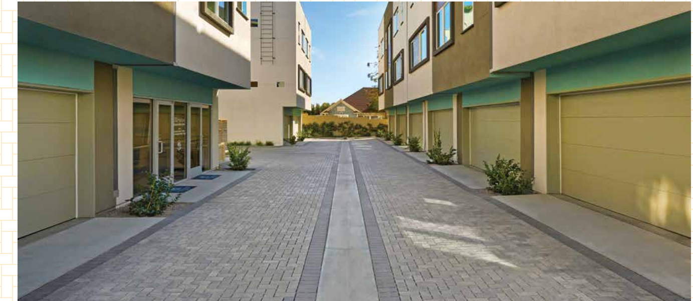
Left and Above: Gray-Charcoal Permeable Holland Pavers installed in a herringbone pattern. The border is solid Charcoal Permeable Holland installed in a soldier course.
