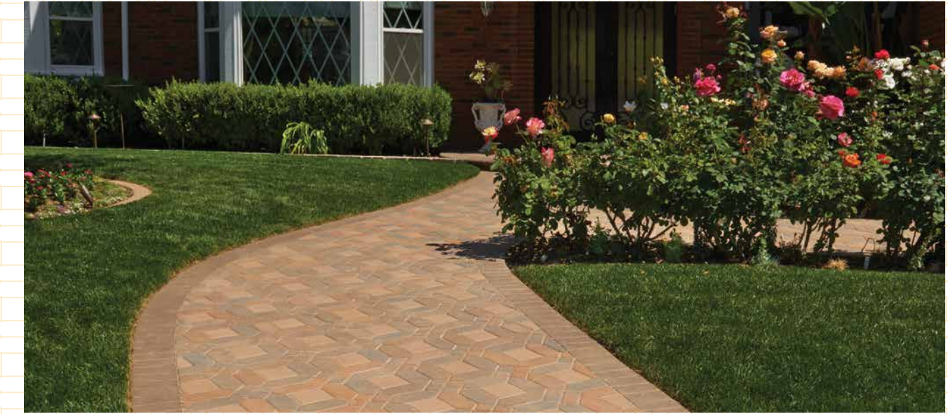
Above: 50/50 field mix of Cream-TerraCotta-Brown and Cream-Brown-Charcoal Symetry and solid Cream 6x6 installed in a Venetian parquet pattern. Border is solid Brown Holland stone in a soldier course.
